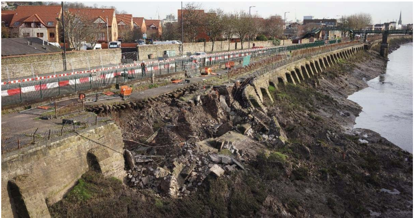
Figure 23: Photo showing the collapse of the riparian wall on Cumberland Road in 2019
